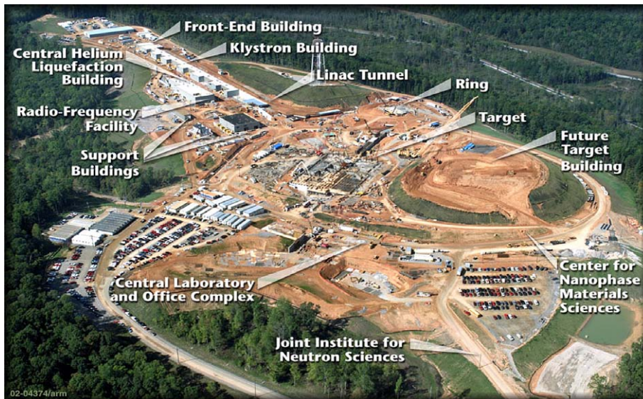
Fig. 2. Progress of the SNS in September 2002. Site excavation, and building construction (labeled) are shown. The foundation for the target building can be seen.
